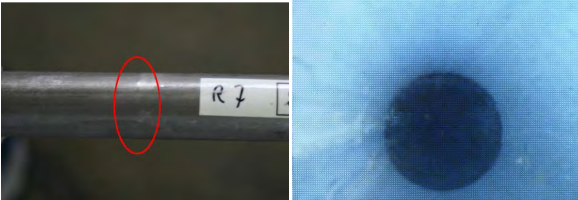
Figure 10: Marks of a mandrel break: The inner diameter changes abruptly. Left: View from outside, right: The inside at this change, seen by an endoscope.
